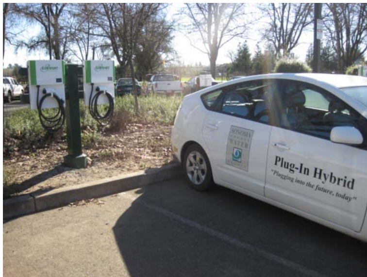
Figure 20: EV charging stations at Administration Building
